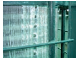
Heavily Corroded HVAC Commercial Units
